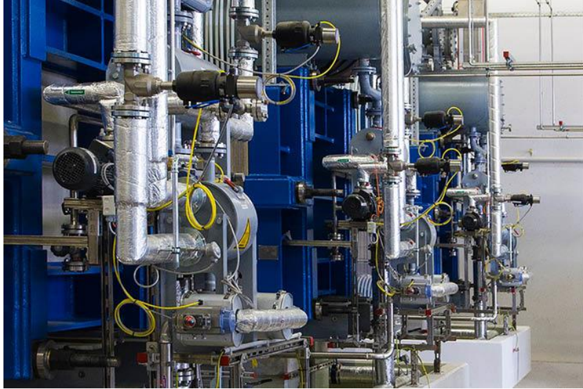
Figure 14.2: three electrolyzers in parallel
